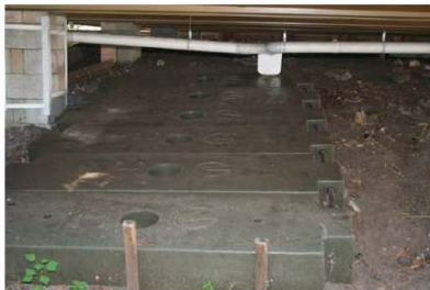
HOG modules bedded into the soil under the transportable classrooms, store 2340 litres (618 gallons) for drip irrigation of surrounding grounds.
